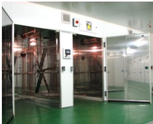
C192 Chick Master Hatcher with stainless steel internal walls and ceiling
